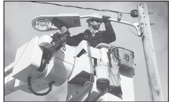
NHEC Conway District Lineworker Ben Mills installs a new LED streetlight in North Conway.
