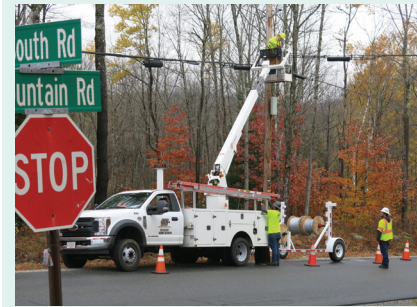
Contract crews installing fiber optic line in Lempster earlier this fall. Service is expected to start this month.
