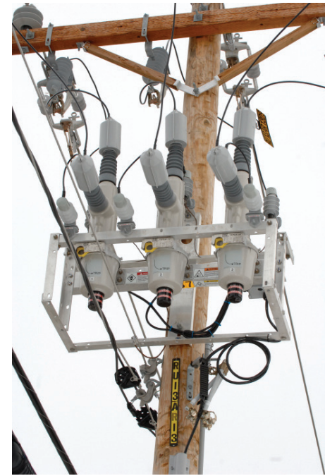
Using technology like this Viper recloser, NHEC is reducing the time it takes to restore power.
