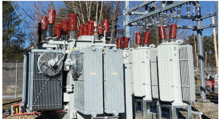
The new NHEC substation in Barnstead nearly triples capacity and features enhanced monitoring tools that allow it to detect and remove abnormal conditions on the system.
