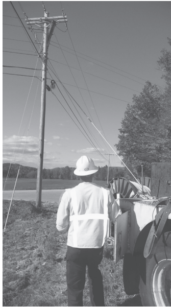
Secured to a tow rope, fiber optic cable is winched into place during installation last month on Yeaton Road in Plymouth.
